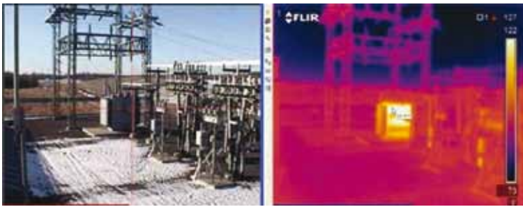
Digital photo and IR image of a substation showing a transformer with excessive temperature.
